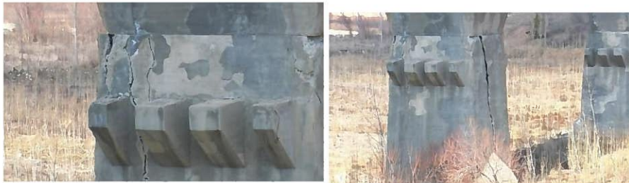
Heavy splitting cracks of piers near foundations
