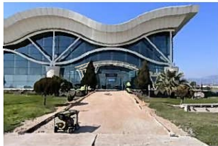
Ground settled around the terminal building at Hatay Airport
