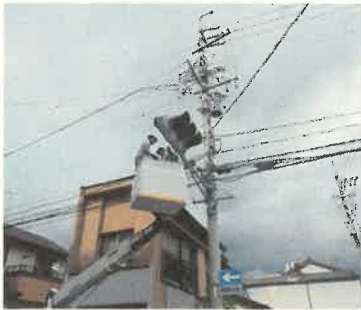
○信号灯器の点検
